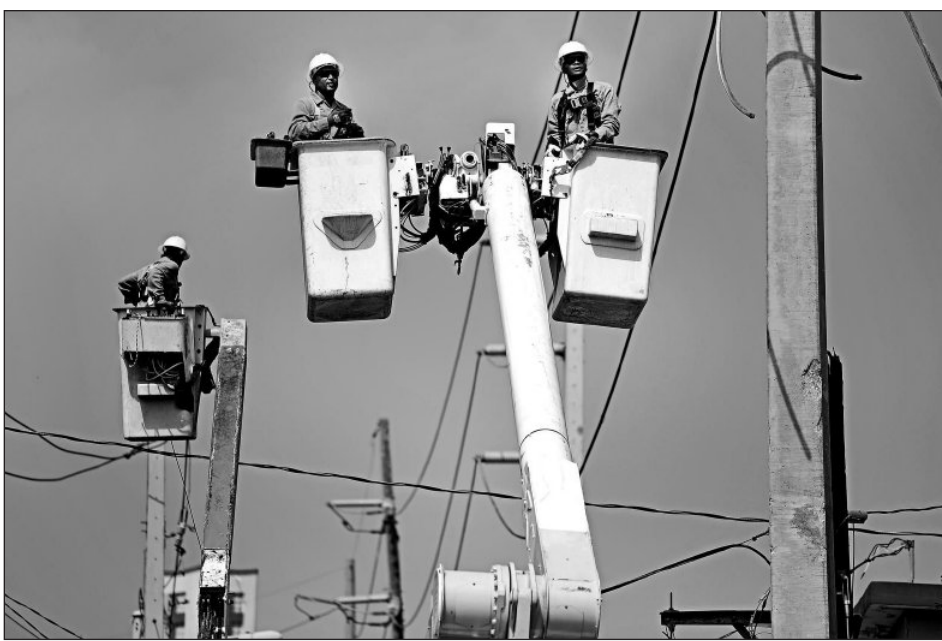
A Puerto Rico Electric Power Authority crew repairs lines damaged by Hurricane Maria. Hundreds of Puerto Ricans remain without power nearly a year after the storm.
