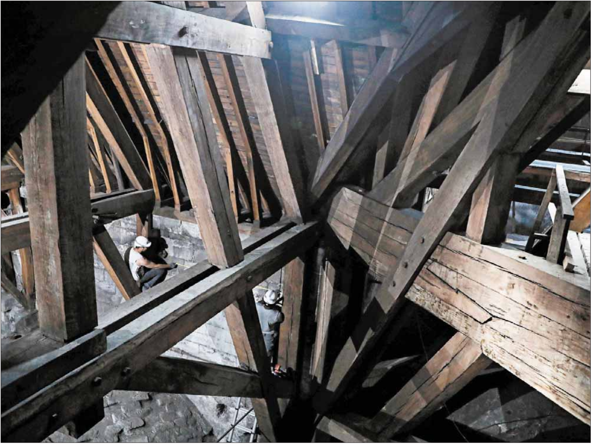
Workers measure a wall as they start restoration work on an old and damaged part of Notre Dame Cathedral on June 26, 2018.
