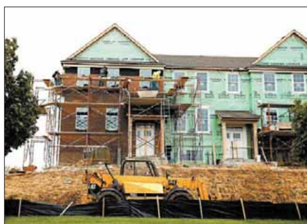
Crews work on town homes in a development in Huntley, which has more than doubled in size since 2000.
