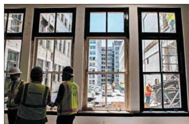
The 11th floor of the building is shown Friday during its renovation by Toronto-based Brookfield Properties. The eighth to 14th floors are being converted to office space and related amenities.
