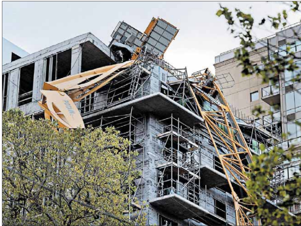
A crane is draped over a building Sunday after Dorian swept through Halifax, Nova Scotia.
